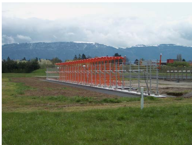
The world's largest and first commissioned Super Wide Aperture Localizer Antenna (278 feet, 85 meters). Watts Antenna Company's Model 201 Localizer Antenna was installed in Geneva, Switzerland, achieving Cat III certification in October 2005.
